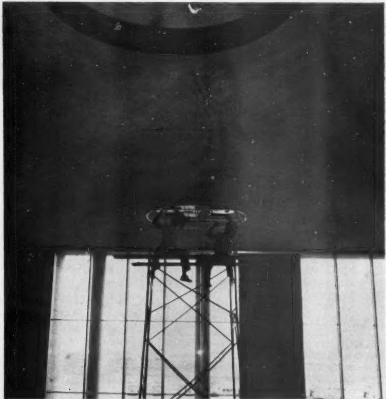
Two workmen of Jack Stone Company are shown atop the 30-foot collapsible steel mobile scaffold used to install the circular lighting fixtures designed especially for mounting in the 30-foot ceiling of Washington National Airport.
